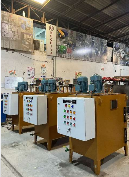
OIL LEAKAGE SYSTEMS
