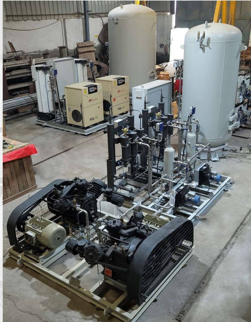
RECEPROCATING & SCREW TYPE - COMPRESSED AIR SYSTEMS WITH AIR DRYERS, AFTER COOLERS
